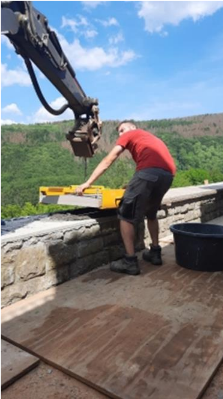
A total of 53 meters of wall coverings made of robust greywacke natural stone were laid. Each of these coverings is custom-made and weighs 60 kilograms. ( Link to high-resolution photo)
